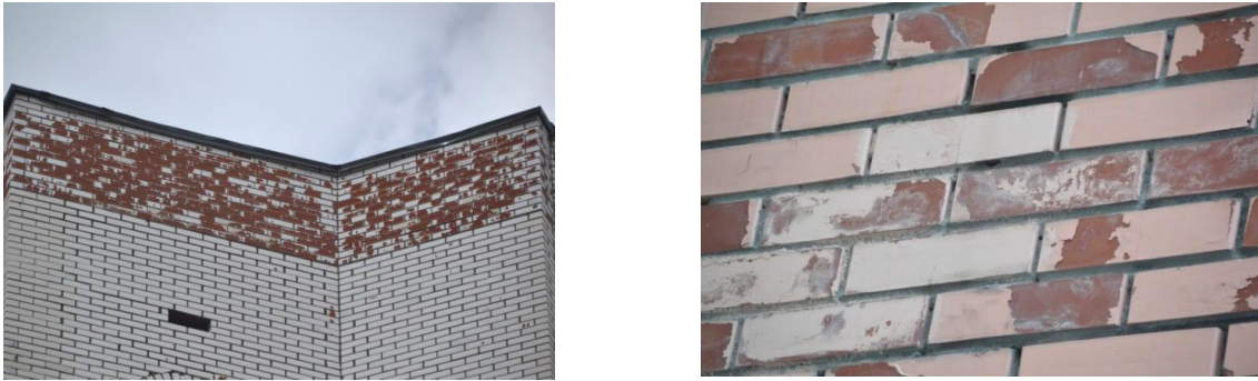
Fig. 1. Destruction of powder paint on the parapet of a residential building (a), peeling of paint from the surface of ceramic bricks (b).
