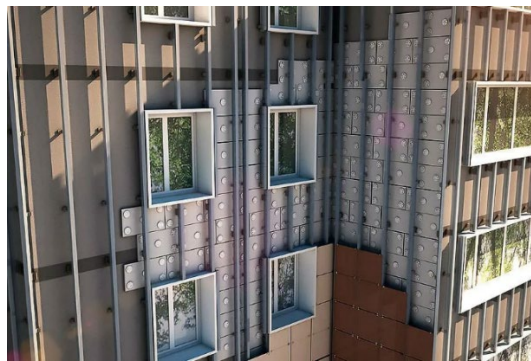
Fig. 3. Configuration of the load-bearing frame of a façade system with vertical profiles.
