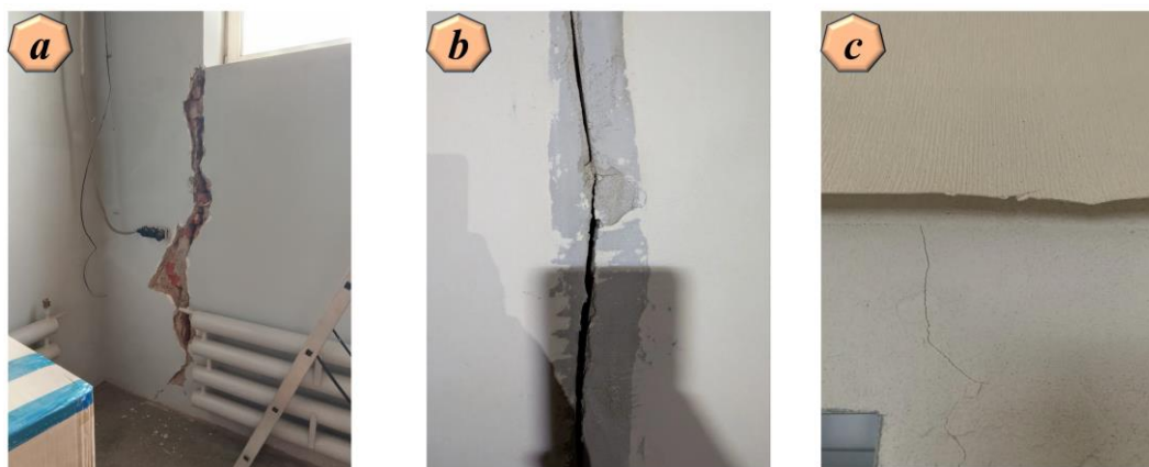
Fig. 1. Typical cracks observed in building walls constructed from different materials: (a) brick masonry; (b) reinforced concrete; (c) foam concrete.
